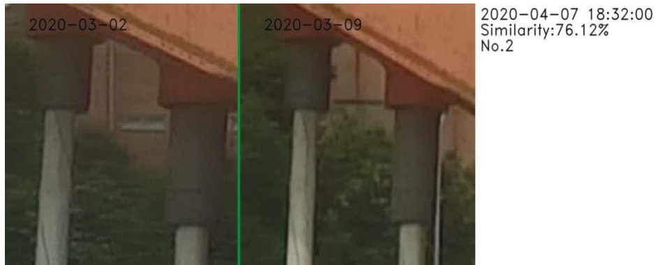
Figure 11 The result includes the bridge node number, the pictures of different days and the similarity of the comparison.
